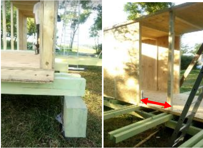
Fig. 22 The installation of floor and wall panels filled with Airium material. Each panel was sized to fit in between base double-beams.
