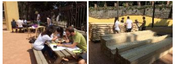
Fig. 10 The group works at the design stage and the decision of timber cut required to build the structures.
