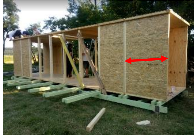
Fig. 20 The installation of nine frame units and wall panels filled with Airium material.
